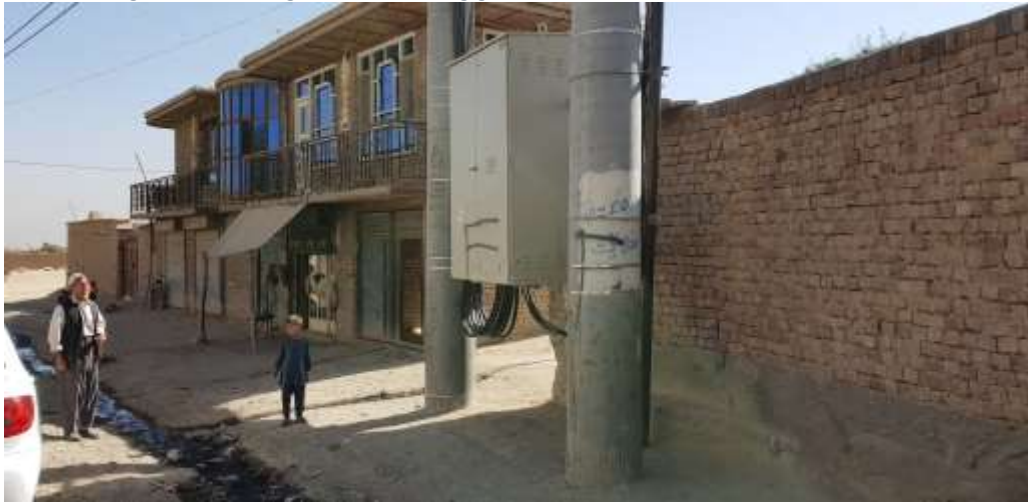
Figure 18 Admiring the new, working grid box in Kata Bolandi, Dasht-e-Barchi, Kabu
