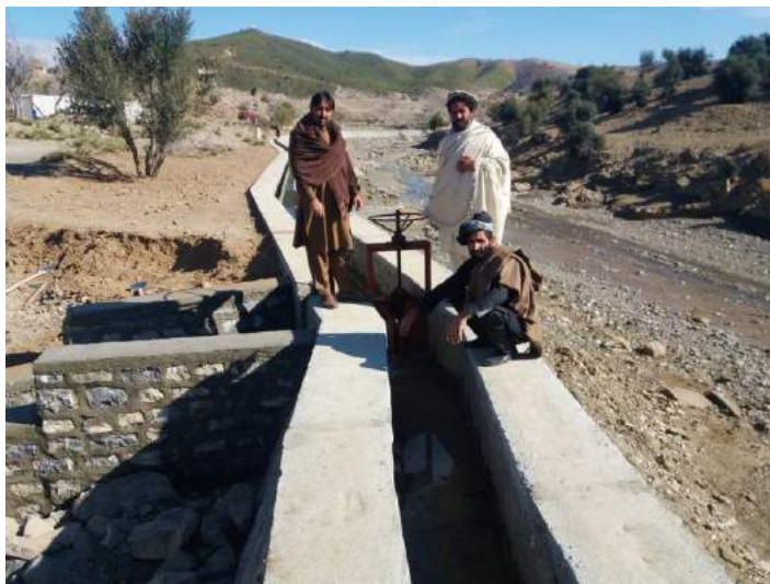
Photo 6. Baghikhail Water Distribution Network built with the support of DACAAR after mine action in the area
